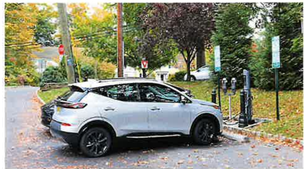
Public Electric Charging Station at The Woodland
