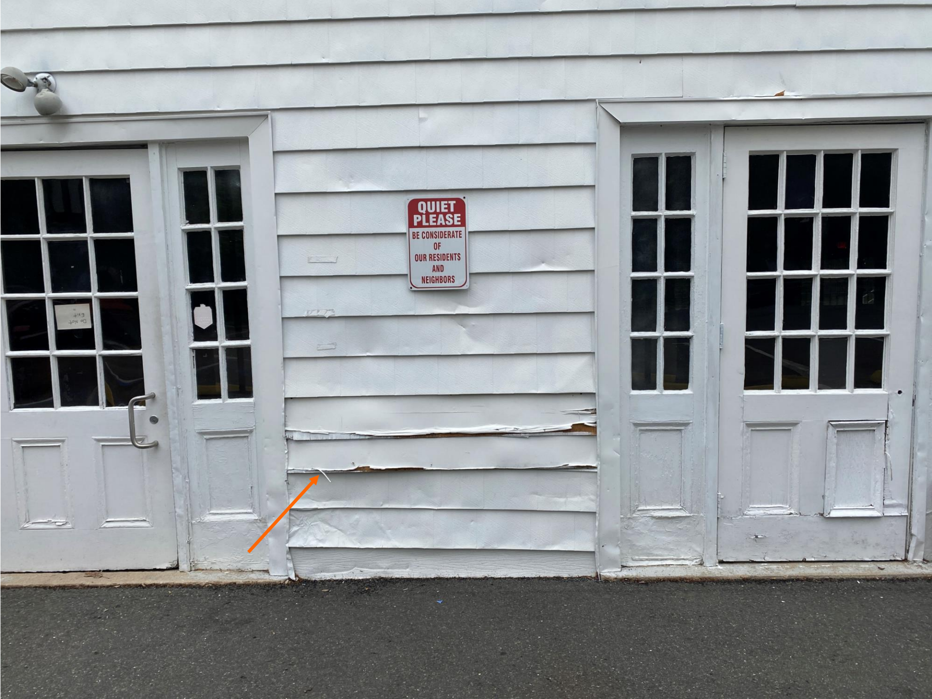
View of replacement siding at the auditorium that looks more like balsa wood.
