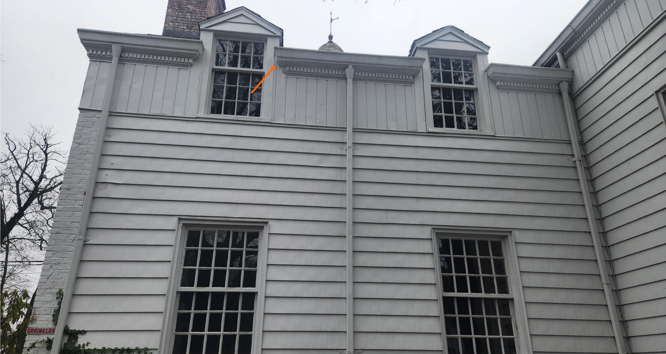
View of the typical detailing of the built-in gutter with some wood rot starting to show.
