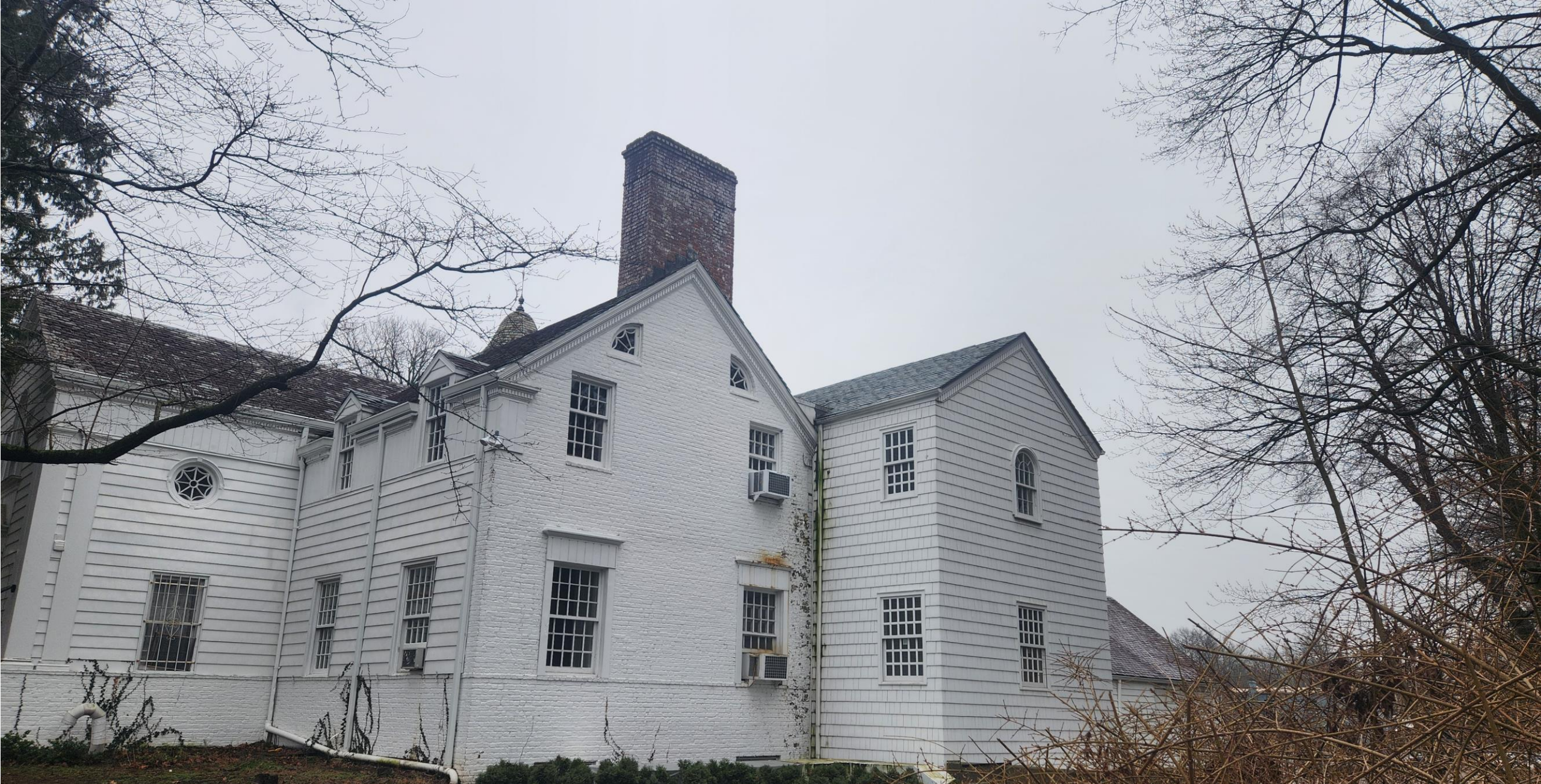
View of the west chimney at the main section roof; the east chimney exhibit similar conditions and both exhibit mortar loss, soiling, and what appears to be paint residue.
